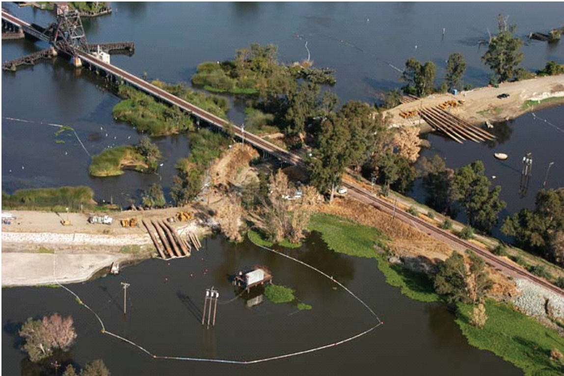
Figure 1.14 Pump out of Upper and Lower Jones tracts (photo) Upper Jones Tract pumps are on the left and Lower Jones Tract pumps on the right of the railroad embankment
