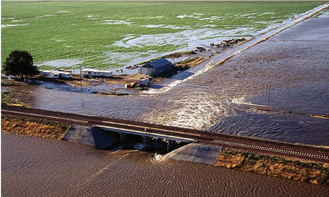
Figure 1.4 Water flowing northward under a railroad embankment from Upper Jones Tract to the Lower Jones Tract (photo)
