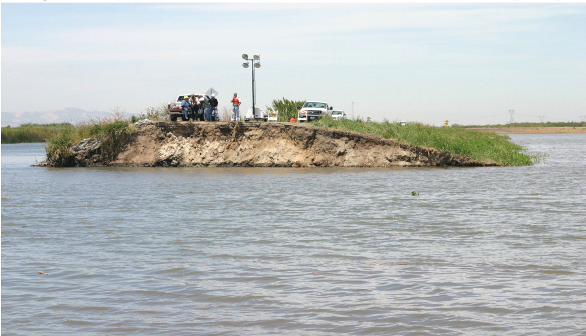
Figure 1.5 Upper Jones Tract levee breach at noon on June 4, 2004 (photo)
