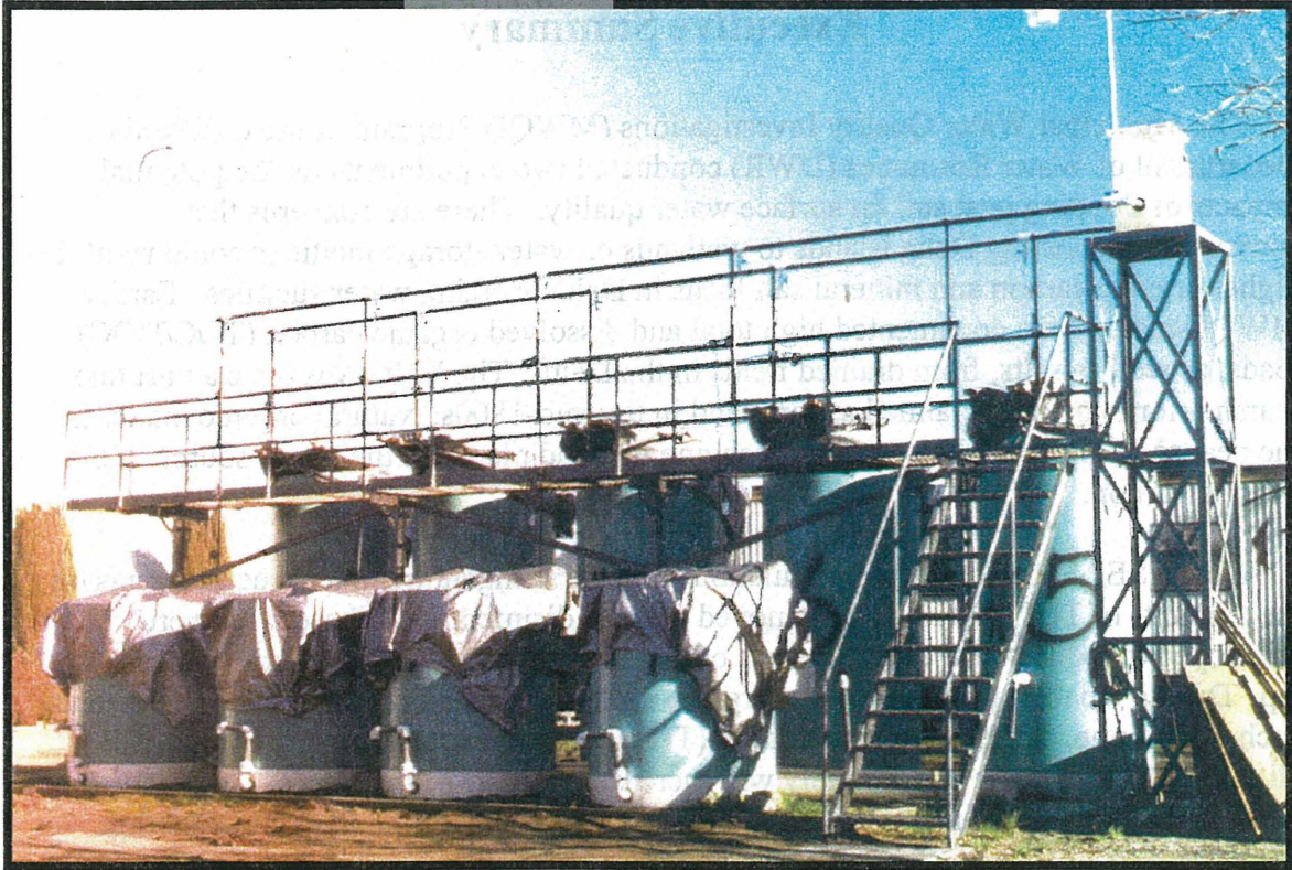
DWR MWQI SMARTS Facility at Sacramento Maintenance Yard in Bryte
